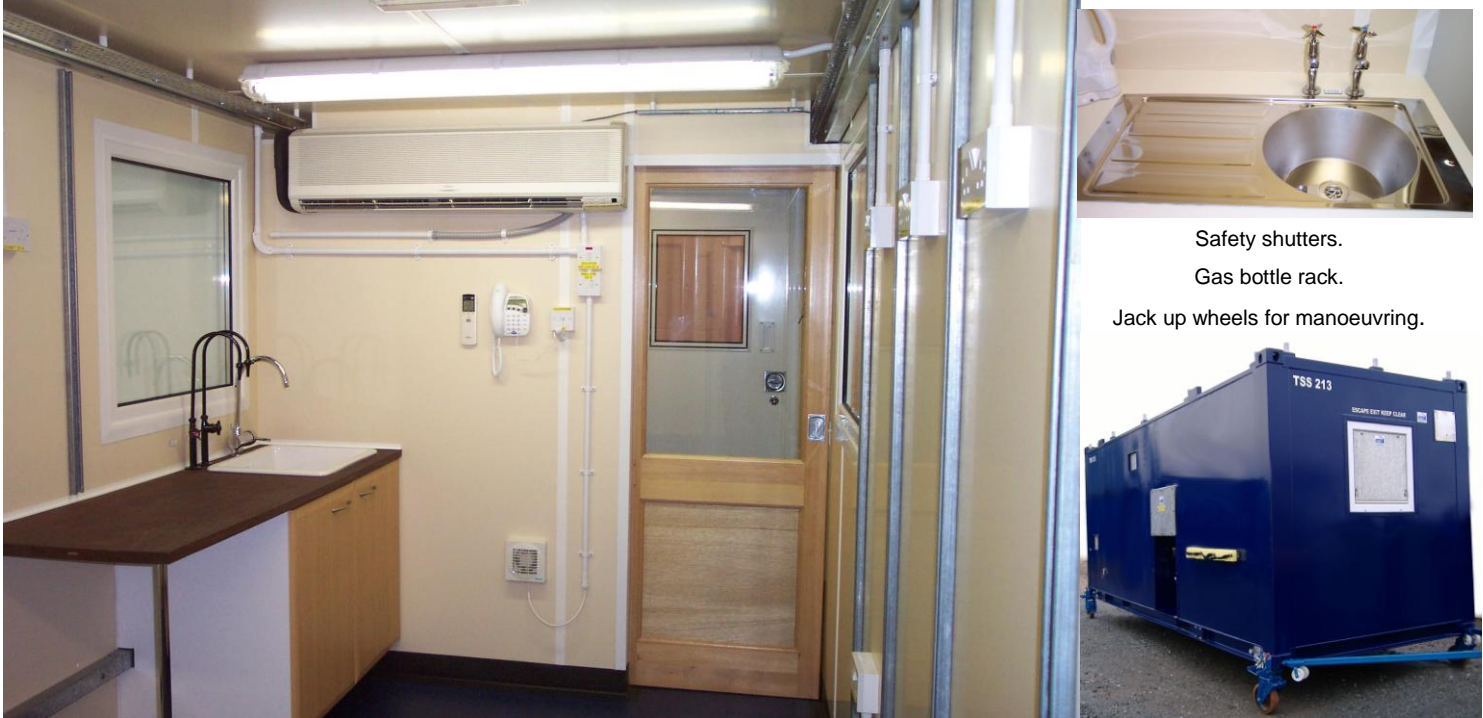
UPS & Hydrogen Generator
